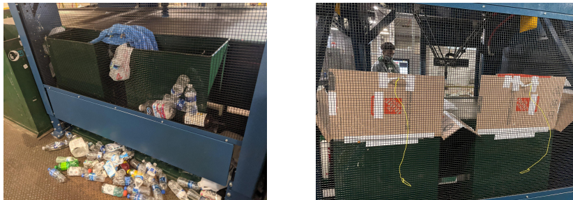
Figure 18: Photographs of clogged material before and after installing the chute shields.
